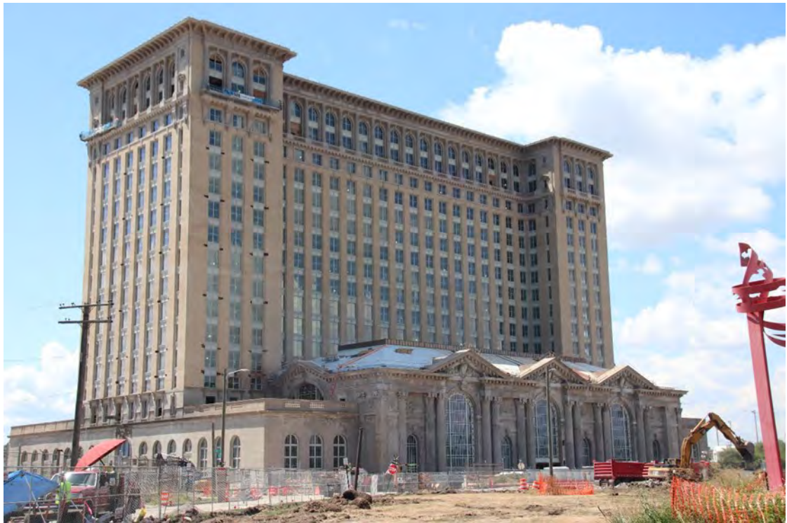
Detroit's Union Depot undergoing restoration. There was an inner and outer chain link fence.
